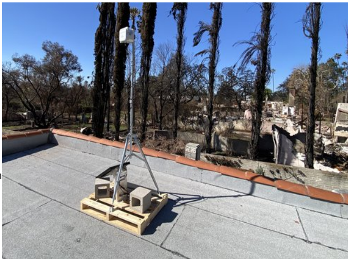
A PHOENIX air quality monitor is mounted on a building in the aftermath of the Eaton Fire. The effort to provide air quality data to the community was rooted in local participation. Credit: Haroula Baliaka
