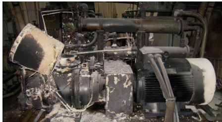
Small-Scale, Isolated Fire Event (Compressor) 5
