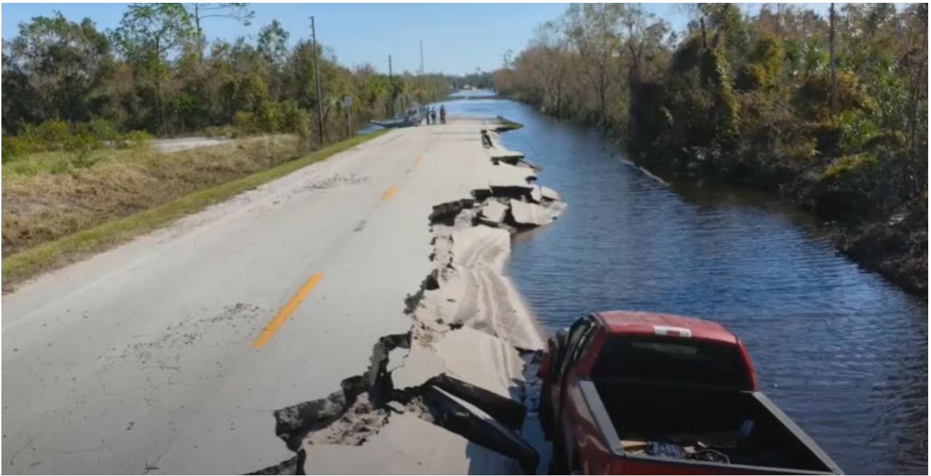
Figure 19: Significant roadway damage in DeSoto County along the Peace River 91
