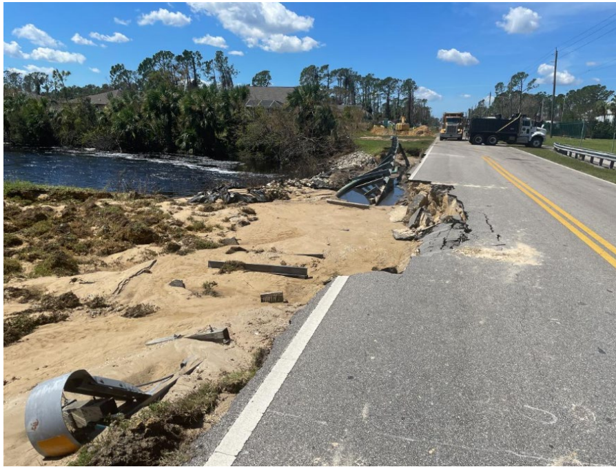
Figure 17: Roadway damage and partial washout near the Myakka River in North Port, Florida 89
