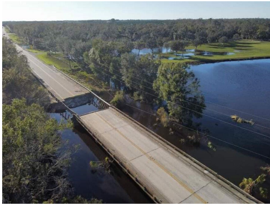
Figure 35. A portion of the Highway 64 bridge near Pioneer Park in Hardee County collapsed due to Hurricane Ian
