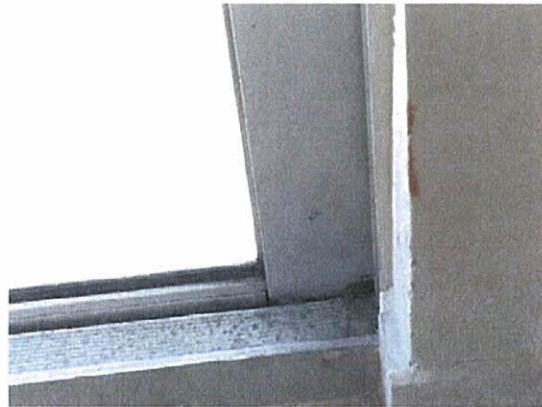
Corrosion stain at kitchen balcony door from possible water intrusion (interior)
