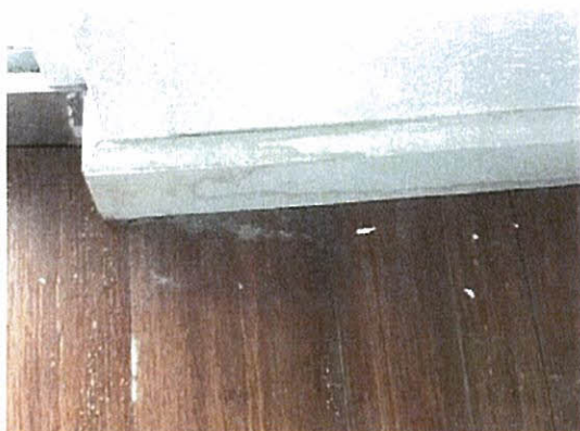
Water stained baseboard and floor
