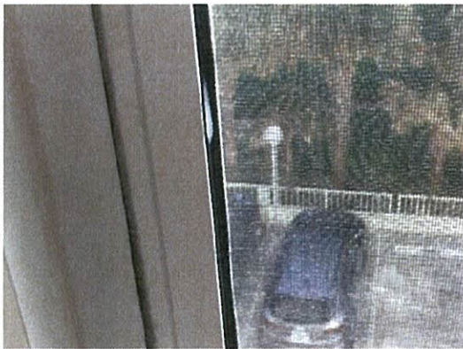
Damaged bedroom window gasket
