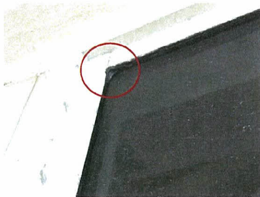
Damaged window gasket at balcony
