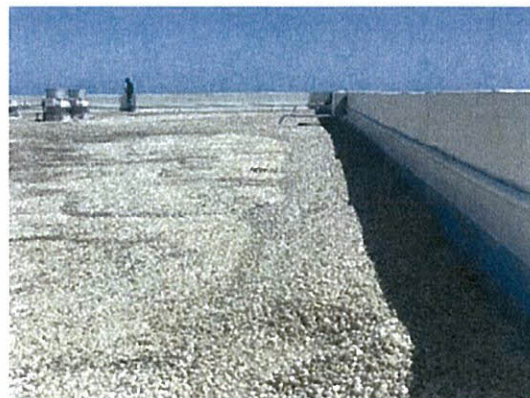
Roof deck gravel accumulation at south side
