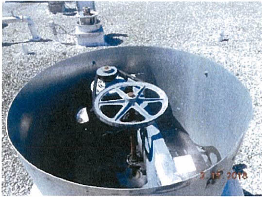
Blown exhaust vent cap
