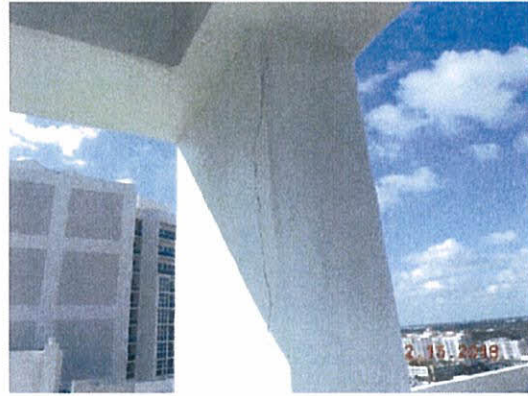
Crack at superstructure column
