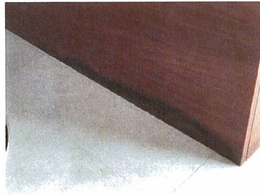
Water stain at base of wood kitchen counter
