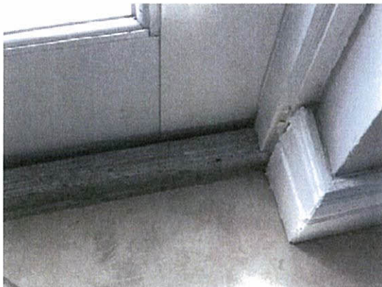
Damaged baseboard at balcony door (interior)
