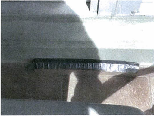
Cracked window sill at balcony window between base and wall (exterior)
