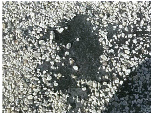
Deteriorated roof membrane panel
