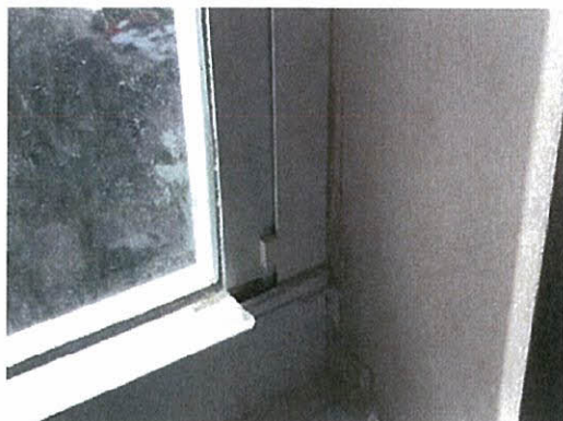
Cracked window frame wall (typical at various locations)
