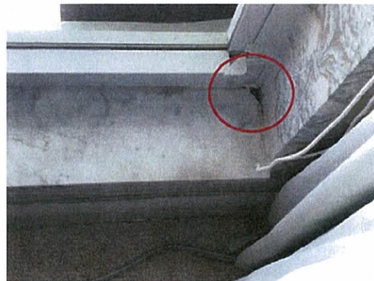
Cracked window sill
