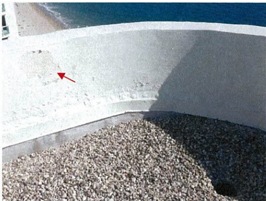
Photo 5.1.1.7 Coating delamination from water infiltration via cracks at wall caused by Irma's combination of intense wind pressures and rain
