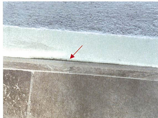
Photo 5.2.2.4 Cracked caulking at balcony wall base trim (exterior) at unit 2008S caused by wind buffeting of tiles due to wind pressures generated during the Hurricane.
