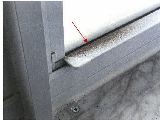
Photo 5.3.12 Sand infiltration accumulated at window lip which enter unit from flexing of windows caused by the wind buffeting that occurred during the Hurricane (PH8N)
