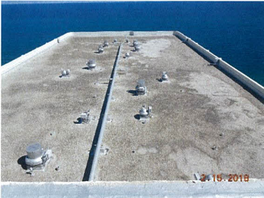
Photo 5.1.2.7 Displaced roof gravel caused by hurricane Irma intense wind gust.
