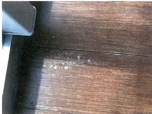
Disjointed and damaged wood floor
