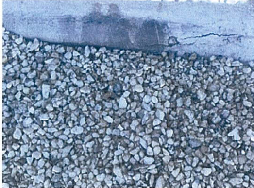
Deteriorated roof membrane
