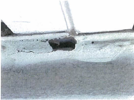
Perforated balcony window caulking
