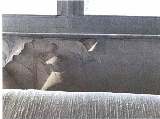
Water intrusion damage along cracked window sill in bedroom
