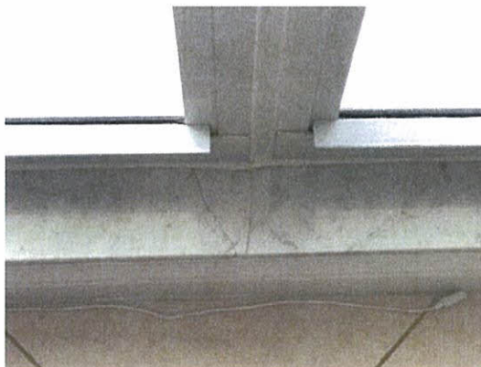
Cracked balcony window sill (interior)
