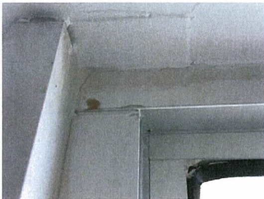
Caulking failure at window frame at the top
