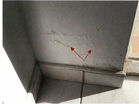
Photo 5.4.1.59 Water infiltration through balcony door caused by the buffeting of doors from Irma's wind pressures.
