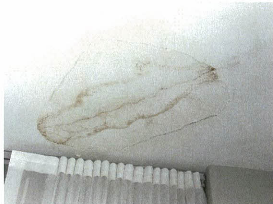
Photo 5.4.1.21 Evidence of water intrusion and damage at ceiling from exterior opening created by the buffeting of windows from Irma's wind pressures.
