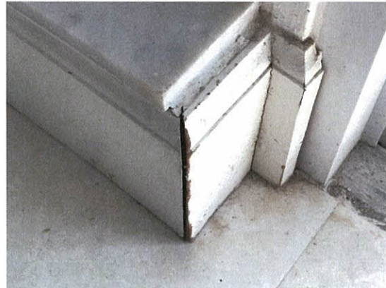
Photo 5.4.1.55 Damaged baseboard from water intrusion through door and window caused by buffeting produced by Irma's wind pressures.
