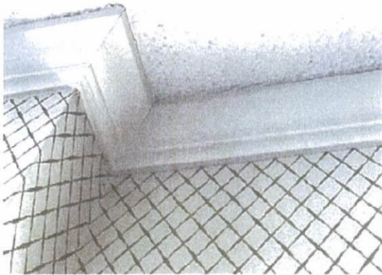
Cracked ceiling board proximate to balcony access. The crack prolongs in length along partition wall and other locations in the living room
