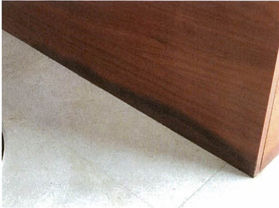
Photo 5.4.1.54 Water stain at base of wood kitchen counter from water infiltration through openings created by the wind buffeting of doors due from Irma's winds pressures.
