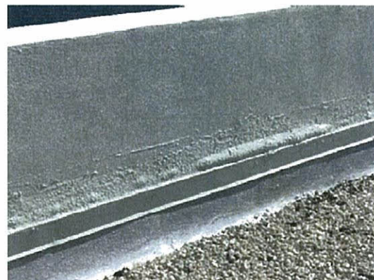
Blister at bottom of parapet wall on the northwest corner of the south tower
