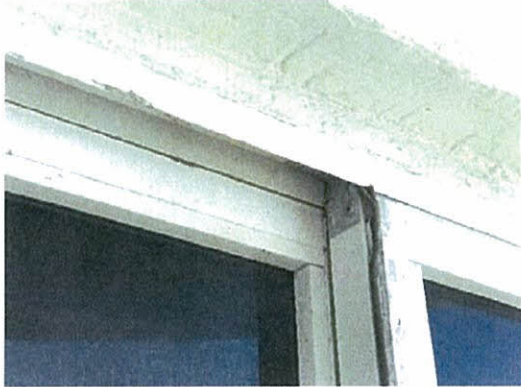
Damaged balcony sliding door weatherstripping
