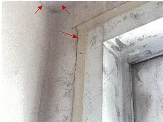
Photo 5.4.1.13 Separation of balcony door caulking at jamb location caused by buffeting of doors produced by the winds during the Hurricane. Also, separations at wall to ceiling interface are indicative of building movement which occurred during the Hurricane.
