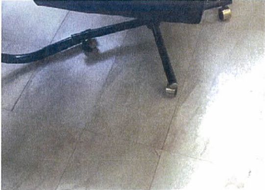
Cracked and disjunct tiles
