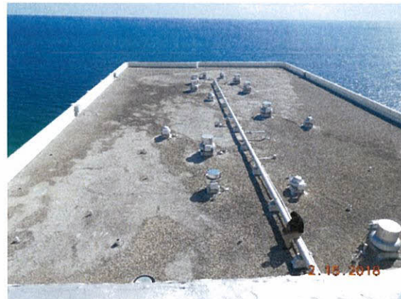
Photo 5.1.1.8 Displaced roof gravel caused by Hurricane Irma intense wind gust
