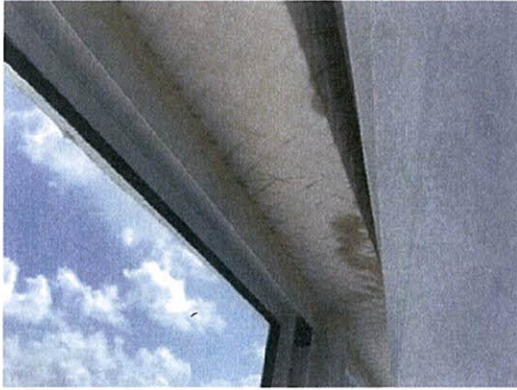
Water intrusion damage and crack at east window header
