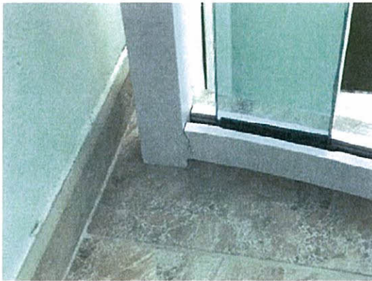
Bottom handrail support cracked
