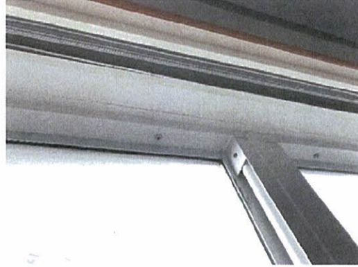
Cracked window header at bedroom
