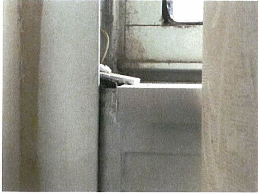
Damaged window frame at living room
