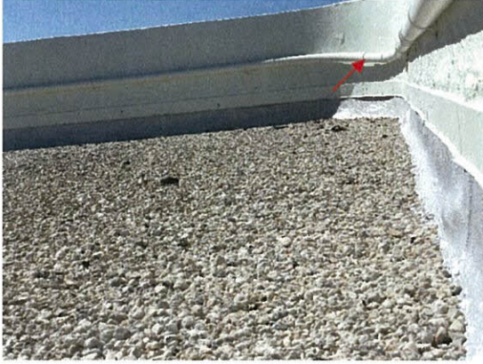
Photo 5.1.2.3 Loose pipe from blown out clamp due to the uplift forces produced by Irma's wind pressures at this location.
