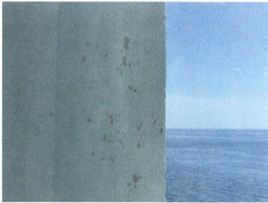
Photo 5.2.1.5 Paint delamination at column caused by Irma's wind pressures at the south tower.
