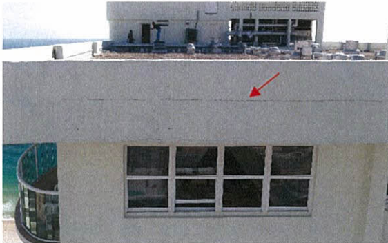
Photo 5.2.1.1 Horizontal crack at parapet wall of the south tower (north elevation) allow water to penetrate exterior and form blisters on the inner face of the parapet wall. Cracks along the building façade were caused by the building movement which occurred during the Hurricane.
