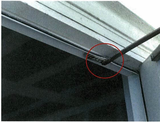
Photo 5.3.5 Bent balcony door frame at top caused by the buffeting of doors due to Irma's wind pressures (1701S)
