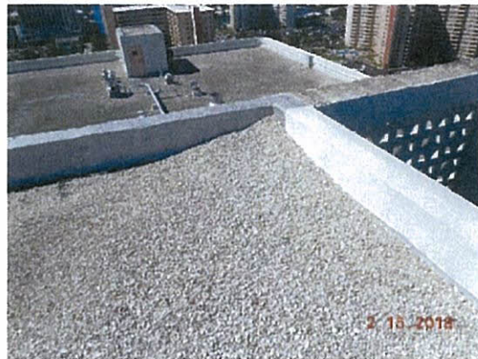
Uneven gravel distribution
