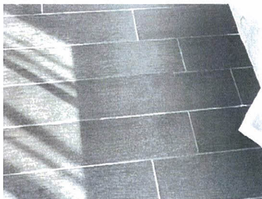
Stained wood floor possibly due to water intrusion
