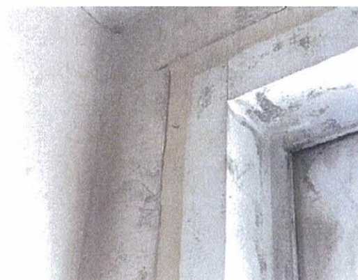
Cracked living room window frame (south side)
