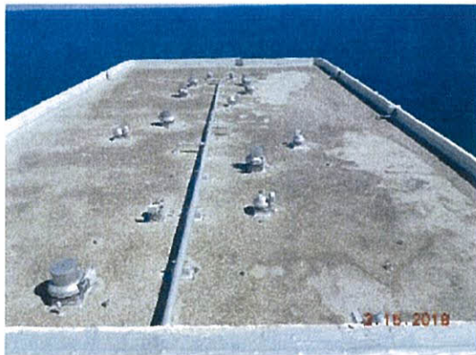
Uneven gravel distribution
