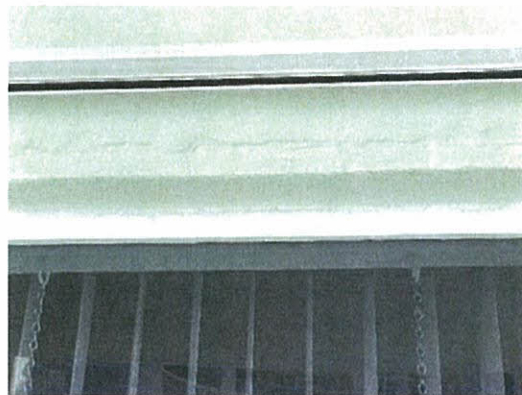
Water bubble atop balcony window header
