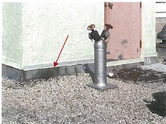
Deteriorated waterproofing system
