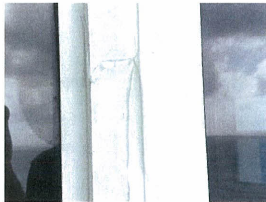
Deteriorated window sealant (exterior)
