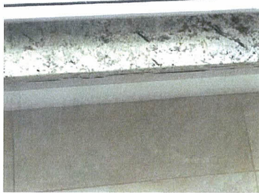
Damaged baseboard below balcony window at living room space
