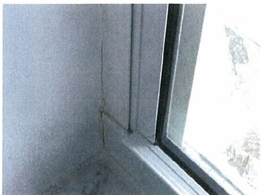
Cracked/Missing window caulking
