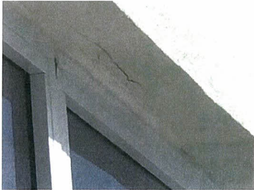
Cracked bedroom window header as seen from balcony (exterior)
