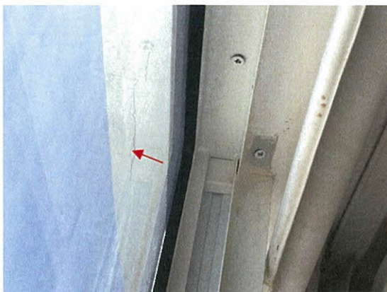
Photo 5.2.1.3 Window header crack caused by the wind buffeting of windows generated by the Hurricane wind pressures allowed water to infiltrate the interior of the unit (at unit 902S). Resident had no issues prior to Hurricane Irma.
