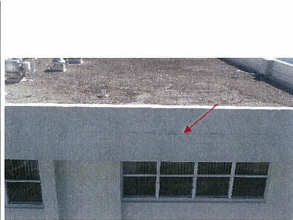
Crack at south most parapet wall of the south tower (north elevation)
