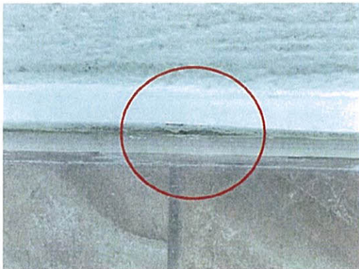
Caulking crack at balcony wall base trim
