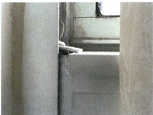
Damaged window frame at living room
