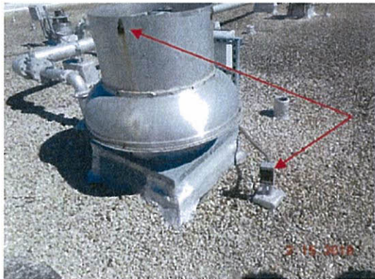
Missing electrical conduit cover/corroded exhaust finish
