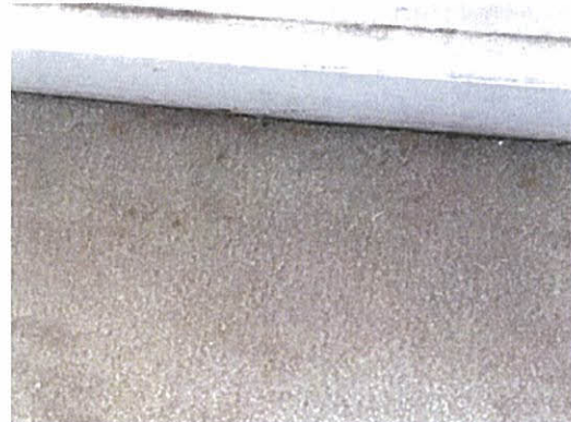
Damage baseboard and spotted corrosion at floor. Carpet was not removed
