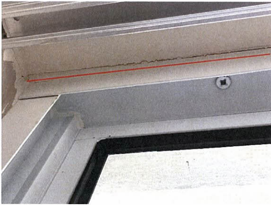
Photo 5.4.1.7 Separation of window board from window sill caused by the buffeting of windows from the Hurricane pressures.
