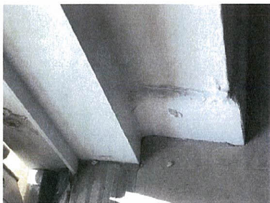
Cracked baseboard and wall finish at balcony door. Signs of water intrusion noticed.
