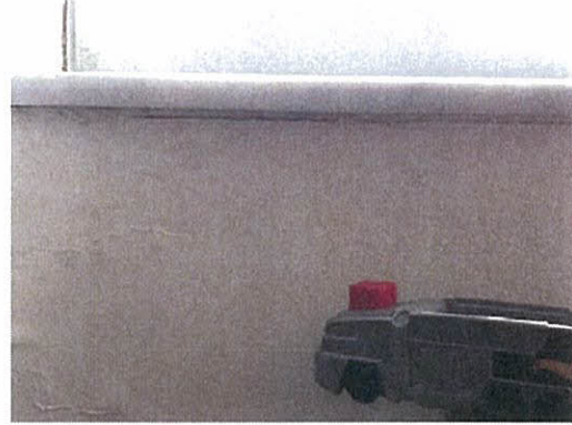
Crack window caulking and water intrusion damage visible at wall below bedroom window
