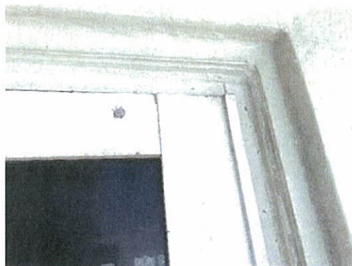
Misaligned balcony door
