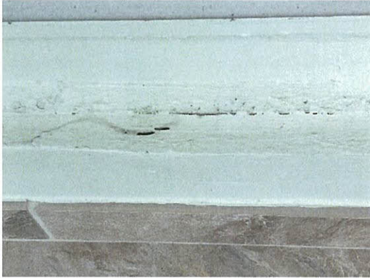
Photo 5.2.2.1 Voids observed at base of windows caused by the wind buffeting of windows produced by the Hurricane wind pressures (at unit 301N)
