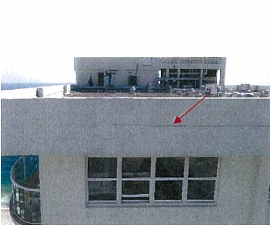
Crack at north most parapet wall of the south tower (north elevation)
