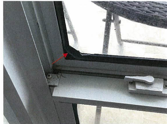
Photo 5.3.18 Displaced window rubber seal caused by the wind buffeting due to Hurricane Irma's wind pressures (2006S)
