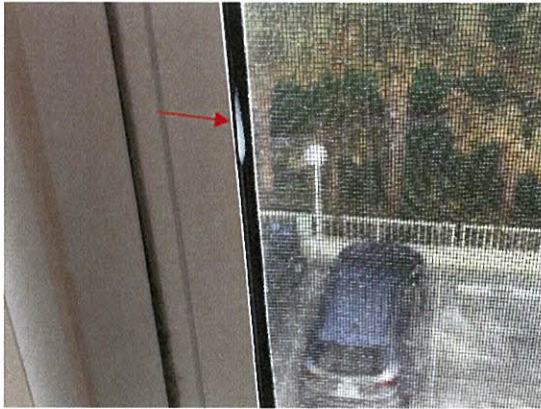
Photo 5.3.13 Displaced rubber seal at bedroom caused by buffeting of windows due to Irma's wind pressures (304S)
