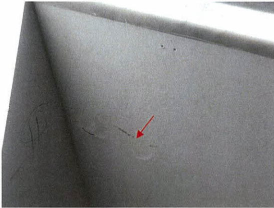
Photo 5.4.1.15 Evidence of water intrusion at wall below window sill which entered through opening at window caused by the wind buffeting due to Irma's wind pressures.
