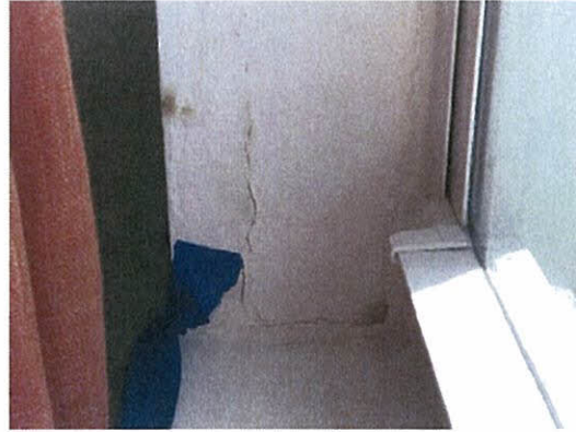
Rust stain and paint failure at wall from water intrusion
