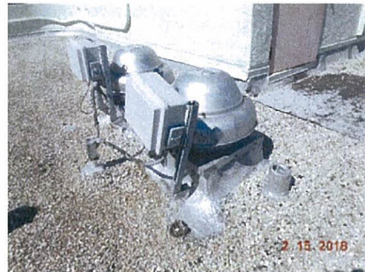
Shifted exhaust electric box possibly due to wind
