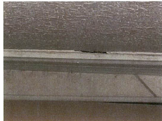
Damage baseboard at east living room wall (unit interior)
