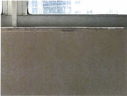
Cracked window sill and missing caulking
