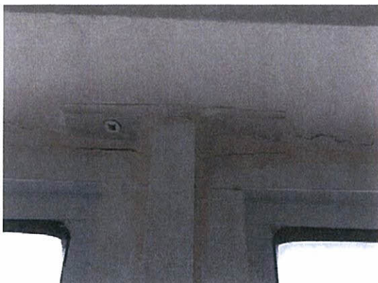
Cracked caulking at mullion connector
