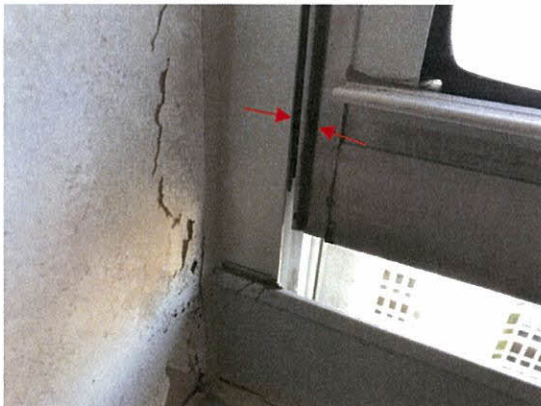
Photo 5.3.15 Racked window frame from buffeting caused by Irma's wind pressures (2106S)
