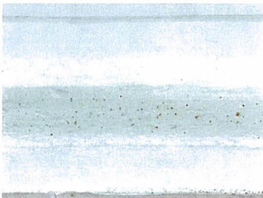
Corrosion at balcony window sill (exterior)
