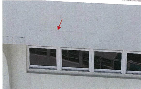
Photo 5.2.1.2 Horizontal crack at parapet wall of the south tower (south elevation) caused by the wind buffeting exerted on the parapet wall generated by Hurricane Irma's wind pressure.
