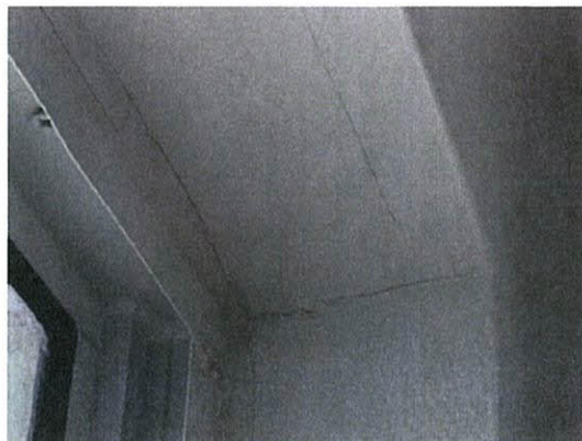
Cracked bottom window header
