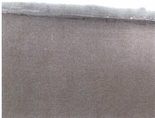
Crack found below window sill at bedroom
