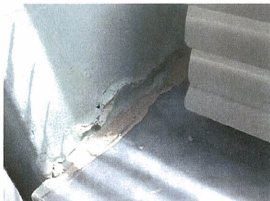
Damaged wall due to water intrusion
