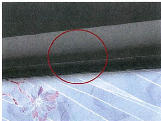
Signs of water intrusion deposited at living room window header
