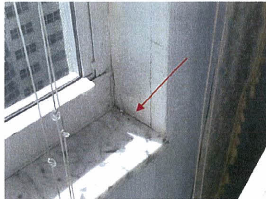
Damaged window frame wall with signs of water intrusion at master bedroom
