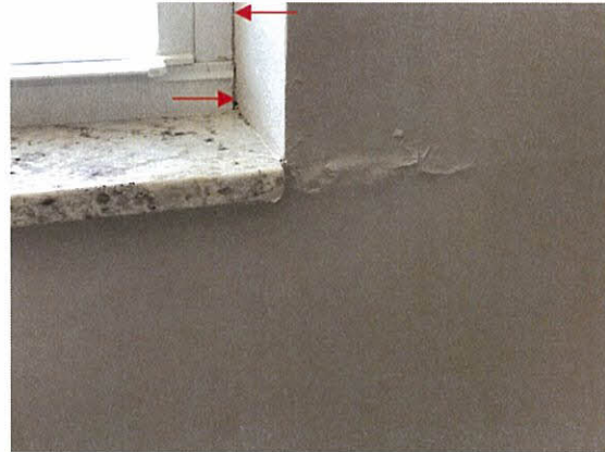
Photo 5.4.1.23 Evidence of water intrusion at window sill level. Also, separation of window frame at jamb location caused by buffeting of windows produced by Irma's wind pressures.
