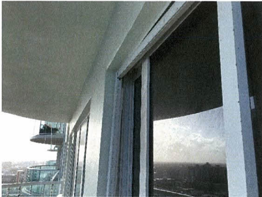
Photo 5.4.1.58 Broken balcony door screener from the wind buffeting of the doors produced by the Hurricane's wind pressures.
