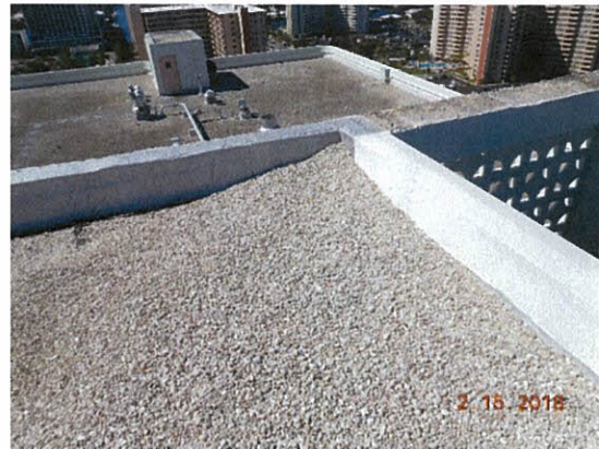
Photo 5.1.2.8 Displaced gravel at machine room roof caused by hurricane Irma intense wind gust.
