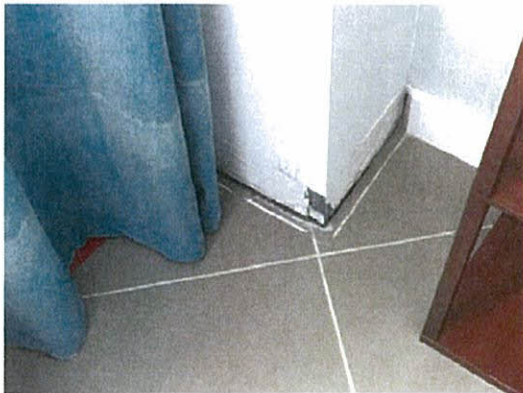
Removed wall baseboard proximate to bedroom window. Water stains visible at curtains
