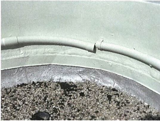
Photo 5.1.1.1 Damaged conduit pipe at roof parapet wall detached by the wind pressures exerted on the building from the Hurricane.
