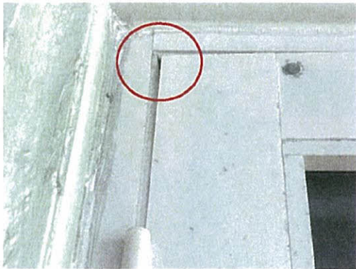
Opening in balcony door weather-strip
