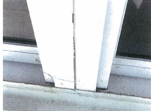
Deteriorated/cracked caulking at balcony door frame
