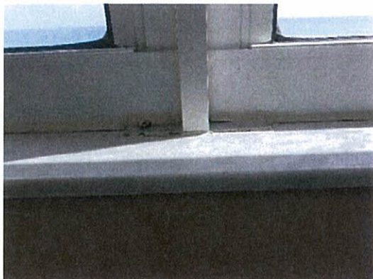
Deteriorated window caulking
