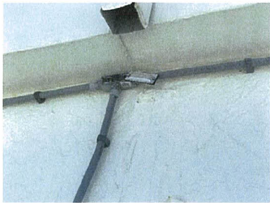
Damaged electric conduit cap
