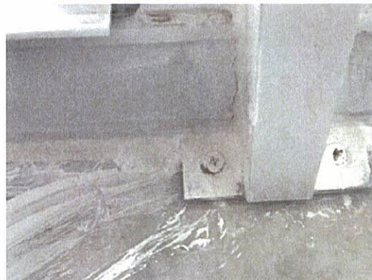
Cracked window base frame
