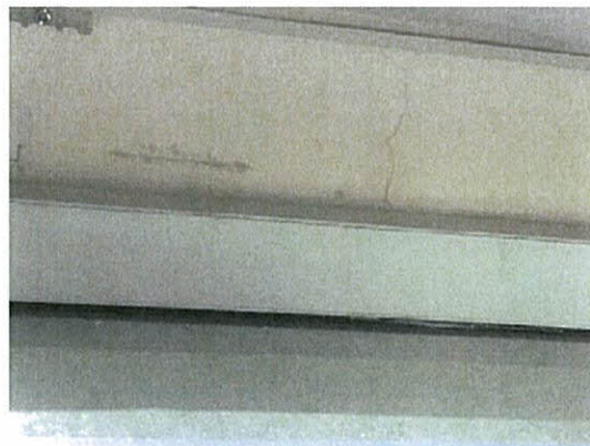
Cracked window header
