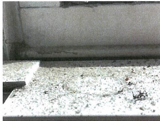
Possible sand accumulation at window corners (interior). Typical throughout all units
