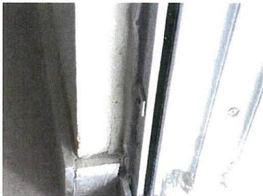
Damaged balcony sliding door frame and baseboard
