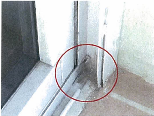
Damaged balcony sliding door and track possibly due to buffeting
