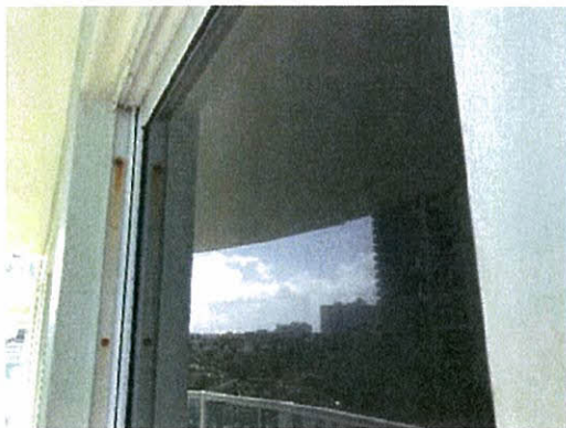
Corroded sliding door screw connectors
