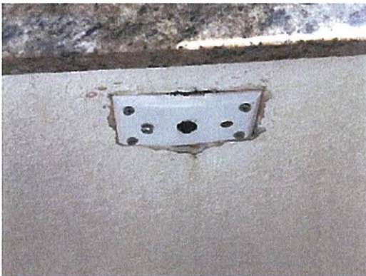
Water intrusion damage at wall below kitchen
