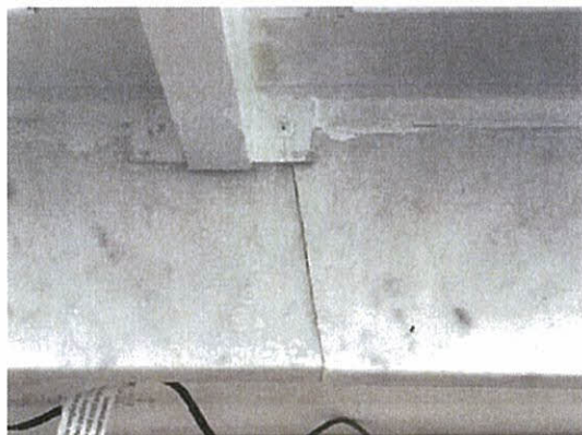
Cracked base finish at window sill
