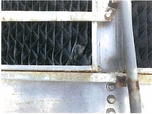
Damaged trickling filter possibly due to wind or debris impact
