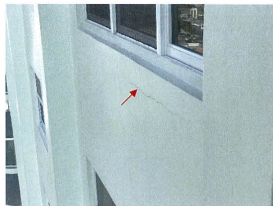
Photo 5.2.1.4 Wall crack at wall below window caused by the wind buffeting of windows produced by Irma's wind pressures allowed water to infiltrate the interior of the unit.
