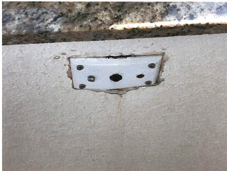
Photo 5.4.1.38 Evidence of water infiltration at wall below kitchen window which entered through opening created by the wind buffeting of windows produced by Irma's wind pressures.
