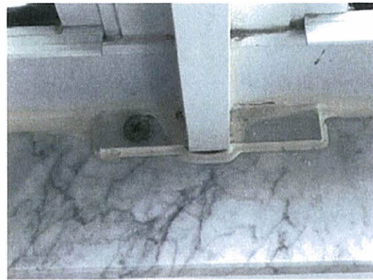
Cracked window base connection caulking
