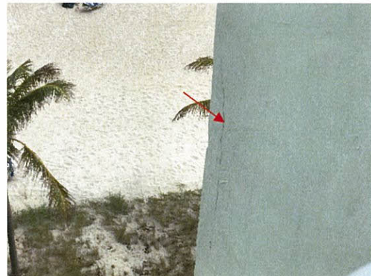
Photo 5.2.1.8 Cracked concrete column as observed from unit 501S caused by the building movement due to Irma's wind pressures.
