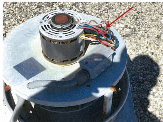
Photo 5.1.2.2 Exposed conduits from blown out fan cover caused by Irma's wind pressure per building staff.
