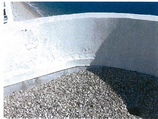
Blister at bottom of parapet wall on the northwest corner of the south tower
