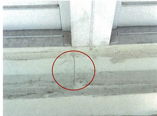
Photo 5.2.2.2 Cracks at base of balcony window (exterior) caused by the buffeting of windows produced by Irma's wind pressures observed at unit 1102N
