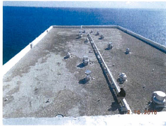
Uneven roof gravel as seen from roof of superstructure
