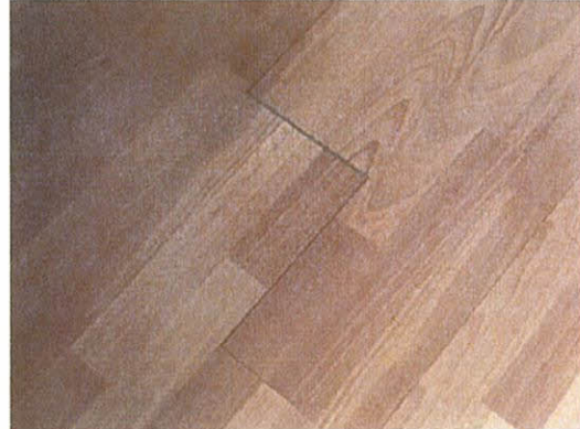
Slightly buckled wood floor possibly from water intrusion
