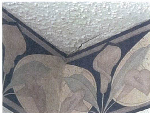
Crack in bedroom ceiling finish typical at spotted locations
