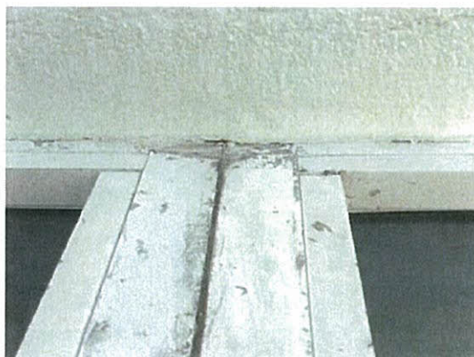
Cracked balcony window header (midspan)
