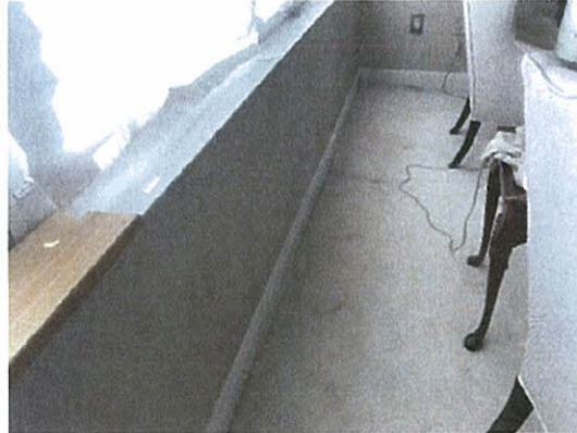
Water intrusion at master bedroom wall and floor
