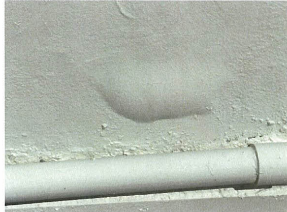
Photo 5.1.1.6 Blisters at parapet wall above the counterflashing from water infiltration via cracks at wall which were caused by the wind buffeting due to Irma's wind pressures.
