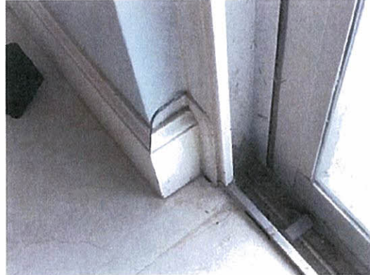
Cracked and detached baseboard at balcony sliding door
