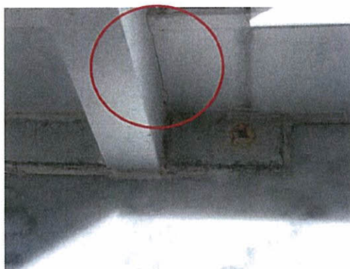
Cracked window frame
