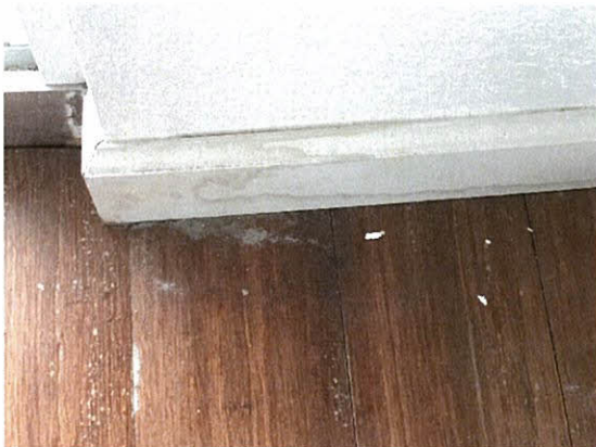
Photo 5.4.1.56 Water damaged baseboard and floor finish from water intrusion through balcony door caused by buffeting produced by the Hurricane's wind pressure.
