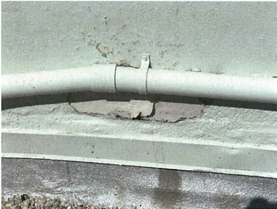
Photo 5.1.2.5 Delaminated paint coat caused by water infiltration through cracks at parapet wall from the wind buffeting caused by Irma's strong wind pressures.
