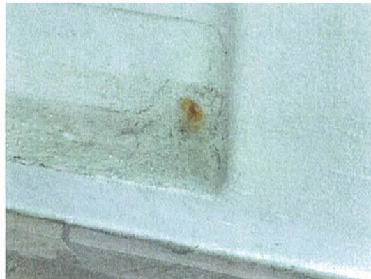
Corrosion happening at balcony window sill
