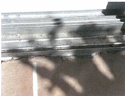
Deteriorated sliding door track caulking
