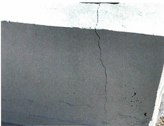
Photo 5.1.1.3 Parapet concrete wall crack on east side of the south tower caused by the wind buffeting to the building envelope generated by Irma's wind pressures.
