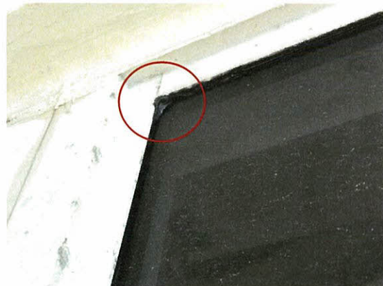
Photo 5.3.4 Damaged window gasket at balcony caused by the wind buffeting of windows from the Hurricane which displaced the rubber seal (gasket) (902S)
