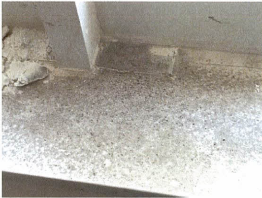
Photo 5.3.11 Sand infiltration at window sill in the bedroom from flexing of windows caused by the wind buffeting which occurred during the Hurricane (204S)
