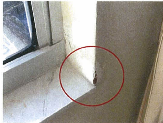
Corroded corner bead at bedroom window possibly due to water infiltration
