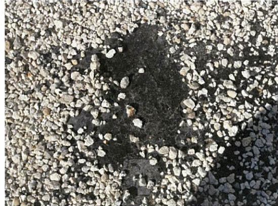
Photo 5.1.1.2 Cracked roof membrane from sun exposure as Irma's winds displaced gravel.
