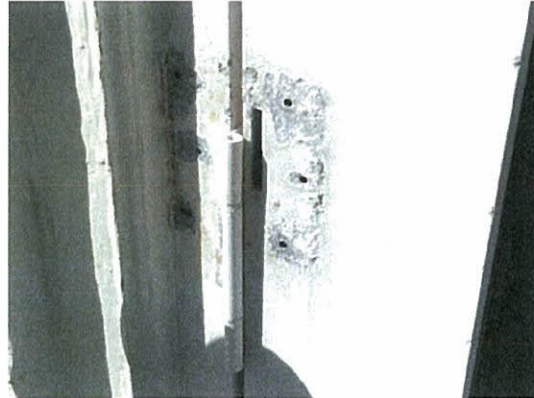
Missing door hinge plate (all 3)
