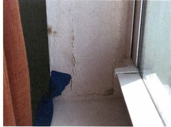
Photo 5.4.1.31 Evidence of water intrusion at window jamb location which entered through opening created by the wind buffeting produced by the Hurricane wind pressures exerted at the windows.
