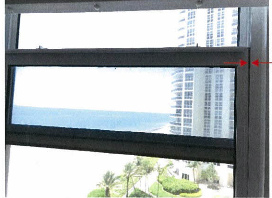
Photo 5.3.18 Racked window frame caused by the wind buffeting of windows due to Irma's wind pressures (702S)
