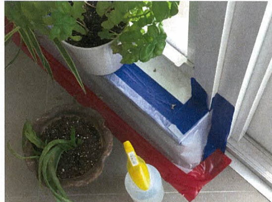
Photo 5.4.1.27 Removed wall section below balcony window sill adjacent to balcony door due to water damage from moisture infiltration.
