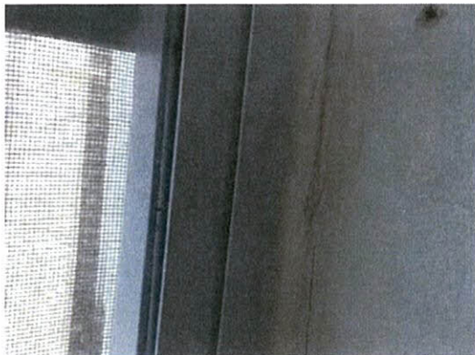
Cracked window frame wall
