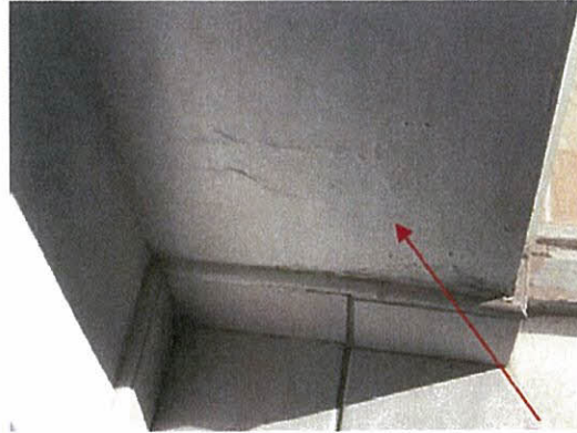
Water intrusion damage at wall proximate to balcony sliding door
