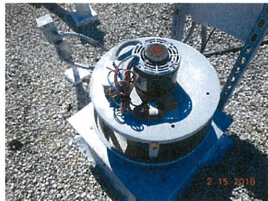
Exposed exhaust electrical wires
