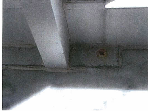
Cracked window frame
