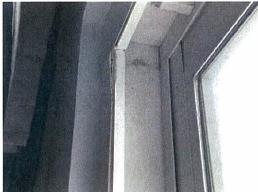
Bent window frame
