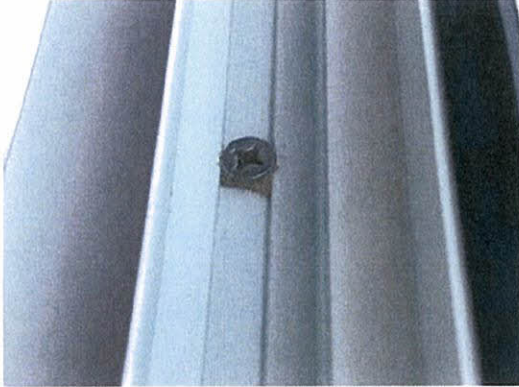
Accumulation of particulates around window semi loose screw (interior)
