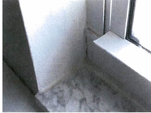
Cracked window frame and wall at bedroom
