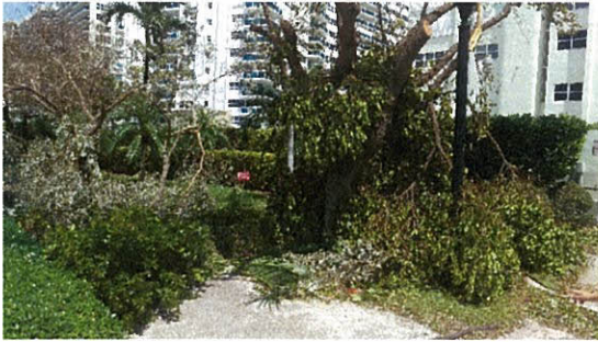
Photo 5.5.1 Damaged landscape at buildings' entrance caused by Irma's wind pressures.
