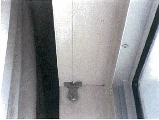
Cracked window header at living room (east side)
