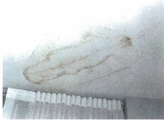
Water intrusion damage at ceiling near east window in the living room
