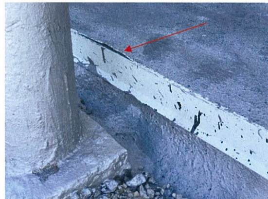
Photo 5.1.2.6 Damaged floor finish above flashing from stresses generated by the Hurricane winds.
