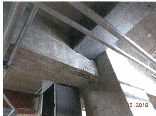
Penetration of roof beam at interior of roof superstructure (not recommended). Typical at both towers
