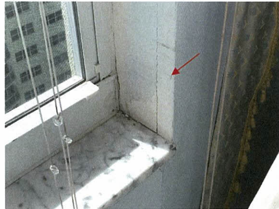
Photo 5.4.1.51 Evidence of water intrusion at window jamb location which entered through openings created by the wind buffeting of windows produced by the Hurricane's wind pressures exerted at the windows.
