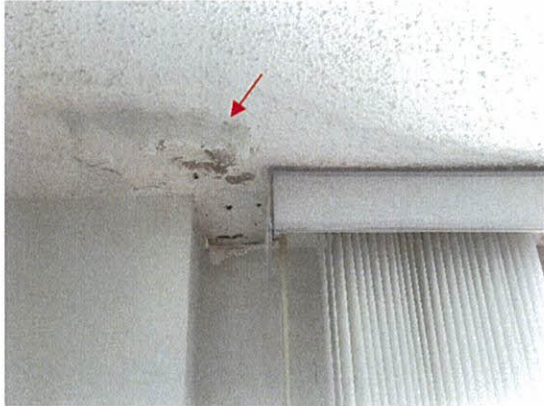
Photo 5.4.1.42 Water intrusion at wall to ceiling interface through window header caused by buffeting of windows created by Irma's wind pressures.
