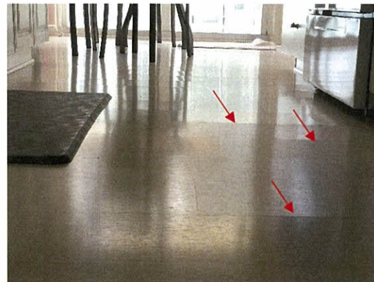
Photo 5.4.1.45 Buckled floor finish at kitchen from water intrusion through balcony door caused by the buffeting of the doors generated by Irma's wind pressures.
