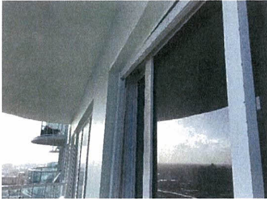
Broken balcony door screener
