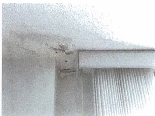
Water intrusion damage at ceiling near balcony window
