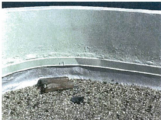
Deteriorated roof deck membrane at angled termination/blister above wall counterflashing
