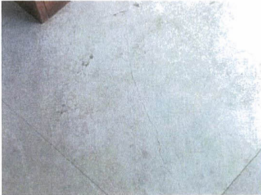
Cracked tile at living room proximate to kitchen counter
