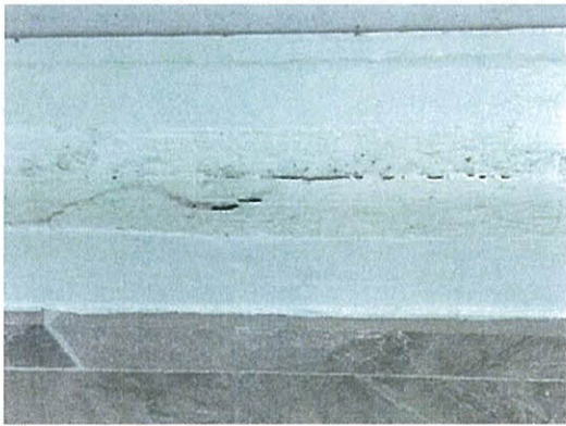
Caulking cracks at base of balcony windows (exterior)
