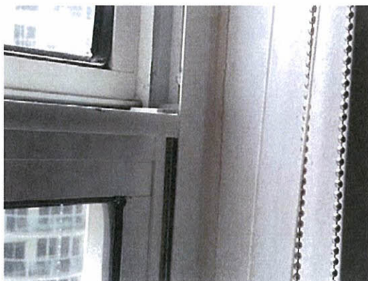
Deteriorated/cracked window caulking
