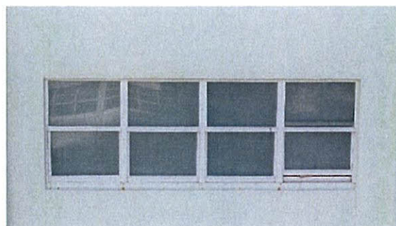
Corroded steel at penetrations left from removal of window shutters
