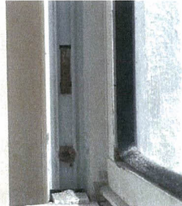
Corroded screws at window frame. Also, cracks observed at frame wall
