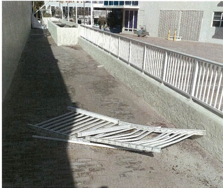
Photo 5.5.4 Blown out aluminum railing from failed post connection caused by Irma's wind pressures (north of tennis court area at north tower).
