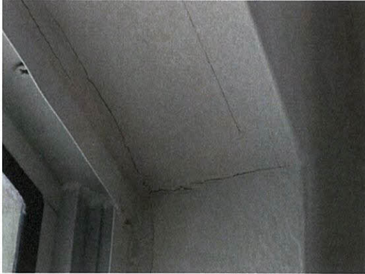
Photo 5.4.1.39 Crack at window header caused by the buffeting of windows from Irma's wind pressures.
