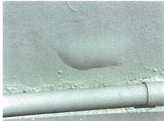
Blister at parapet wall on the southwest side of the south tower
