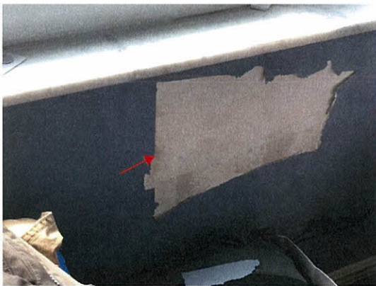
Photo 5.4.1.17 Paint failure from water intrusion through opening at window sill created by the buffeting of windows.
