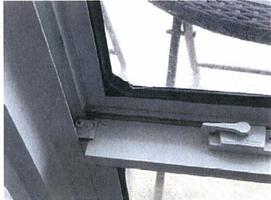
Damaged balcony window gasket
