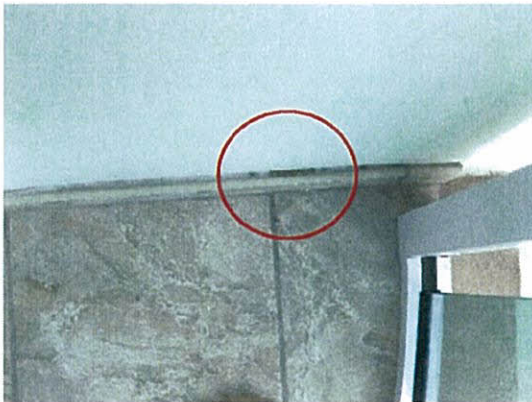
Signs of water intrusion through balcony baseboard
