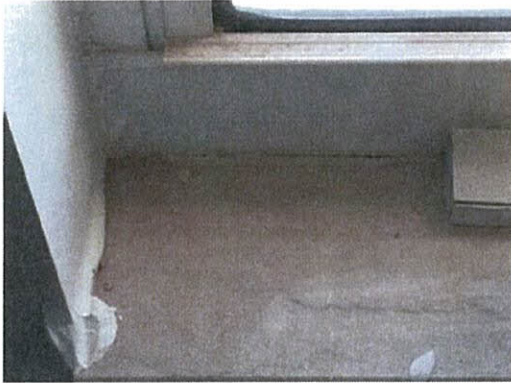
Cracked window caulking at window sill
