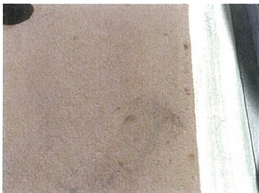
Rust spots at balcony slab (various locations)
