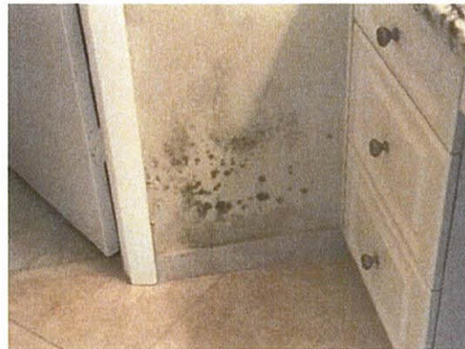
Biological growth found at master bathroom wall
