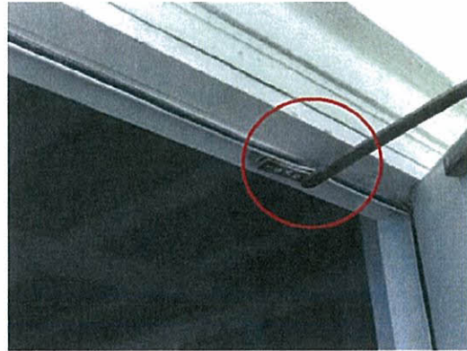
Bent balcony door frame at top
