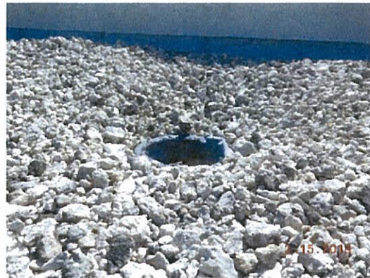
Deteriorated roof membrane panel
