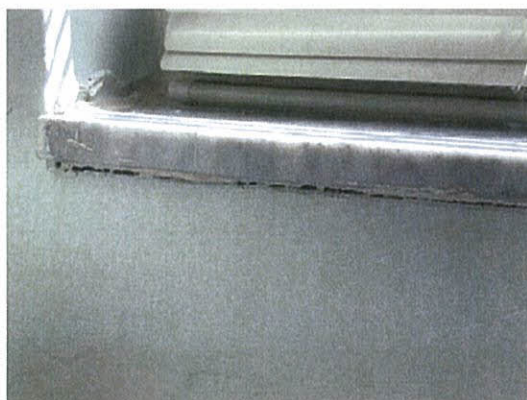
Wall cracked along perimeter of window sill
