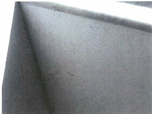
Water intrusion at kitchen wall below east window
