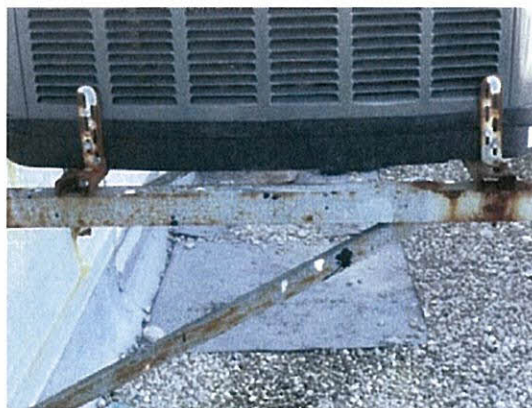
Corroded compressor unit support and connections
