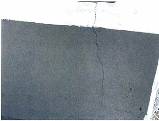
Parapet concrete wall crack on east side of the south tower
