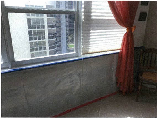
Photo 5.4.1.26 Removed wall section below window sill due to water damage from moisture infiltration.
