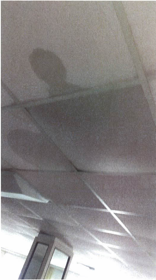
Photo 5.4.2.1 Water damage at lounge area roof that entered through openings created by buffeting of windows due to Irma's wind pressures (south tower).
