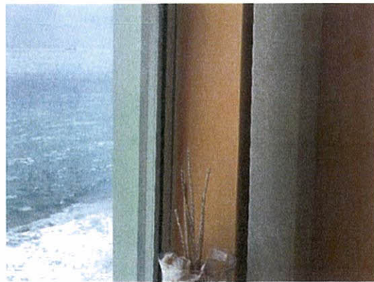
Failed kitchen window caulking
