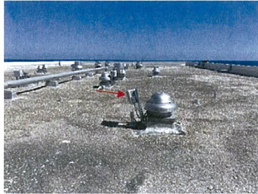
Impacted exhaust electric box
