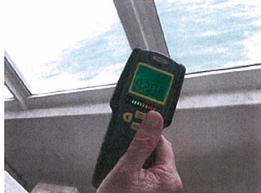
Allocated wall moisture content at corners (windows facing east)
