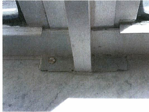
Damaged window bottom connection
