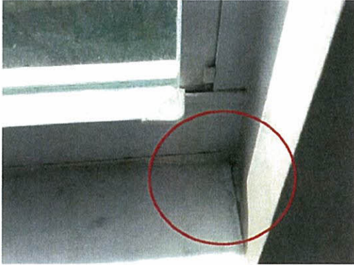
Cracked master bedroom window sill at right hand corner
