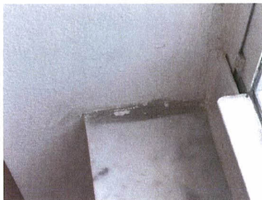
Cracked window caulking
