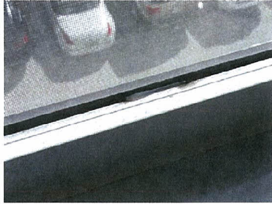
Master bedroom window gasket damaged
