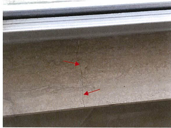
Photo 5.4.1.8 Cracked window board caused by the buffeting of windows due to Irma's Hurricane pressures.
