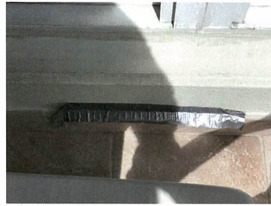
Photo 5.2.2.6 Failed caulking covered below balcony window caused by wind buffeting of tiles due to pressures generated during Hurricane Irma (exterior) (1202N)
