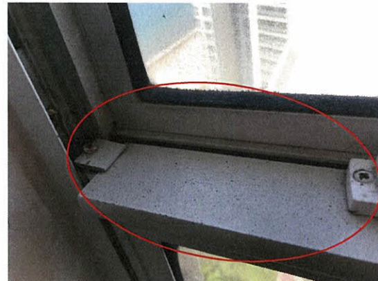
Photo 5.3.16 Sand intrusion through window opening caused by the buffeting of windows generated by Irma's wind pressures. See photo 5.3.15. (Unit 2106S)
