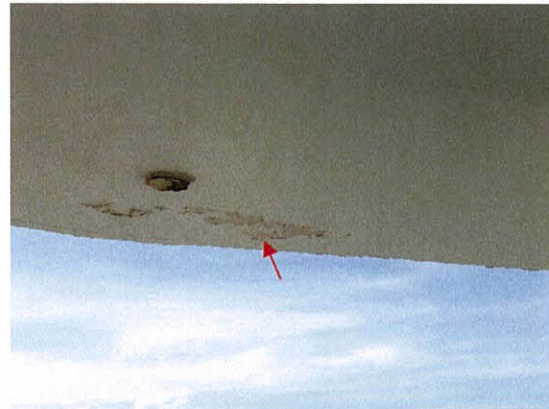
Photo 5.2.1.6 Paint delamination at projected slab soffit caused by Irma's wind pressures (observed from unit PH1S).
