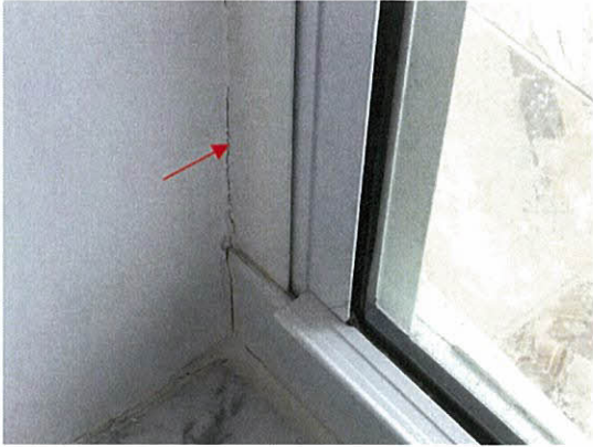
Photo 5.3.9 Cracked balcony window caulking caused by the wind buffeting of windows due to Irma's wind pressures (301N)
