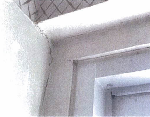
Deteriorated/cracked caulking at balcony door frame
