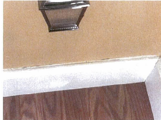
Damaged baseboard possibly due to water intrusion
