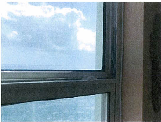
Cracked window frame at living room (east window)
