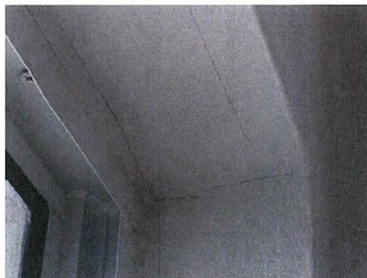
Cracked window header
