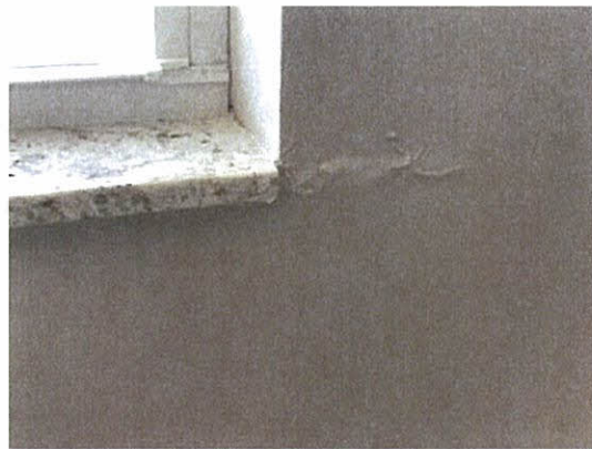
Paint blisters possibly due to water intrusion visible at the east window at window sill level
