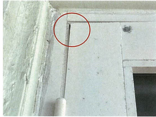
Photo 5.3.6 Separated door rubber seal caused by the wind buffeting at balcony door generated from Irma's wind pressures (1602S)
