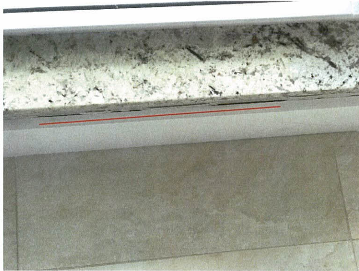
Photo 5.4.1.19 Separation baseboard to knee wall below window sill caused by buffeting of windows produced by Irma's wind pressures.
