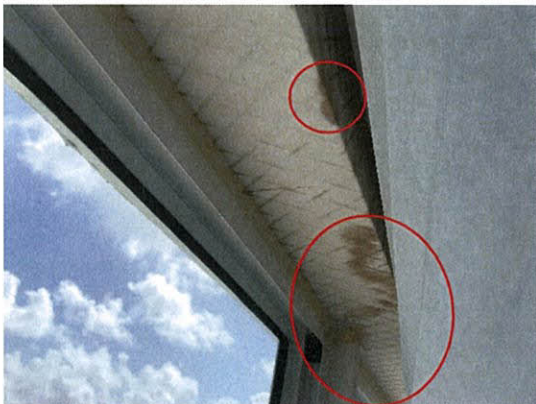
Photo 5.4.1.48 Water intrusion damage at east window header from opening created by the buffeting of windows due to the Hurricane's wind pressures.
