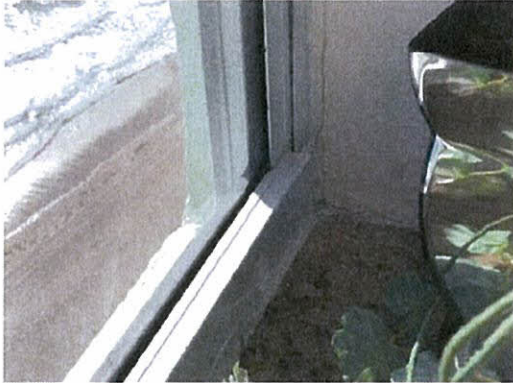
Cracked stucco along window frame at southeast corner near kitchen
